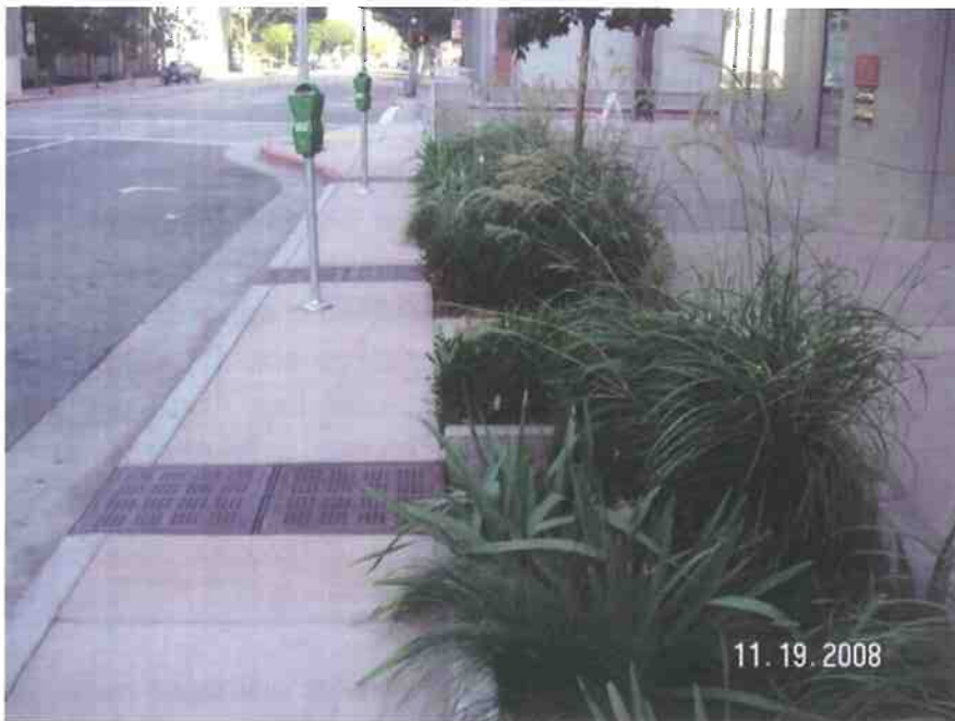
Curb inlet and infiltration basin in Downtown LA--Hope Street and 11th Street.
